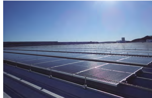
Saitama Factory's assembly plant (2.0 MW)
